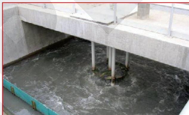
Grit and sand removal tank
